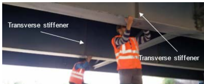
Fig. 7. Placement of strain gauges near transverse stiffeners.
